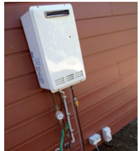
An instantaneous gas hot water system
