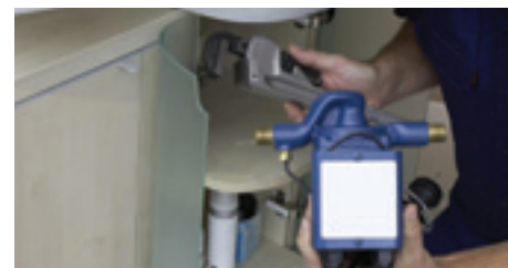
Water recirculation devices are usually located under kitchen or bathroom sinks
