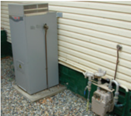
An example of a storage gas hot water system
