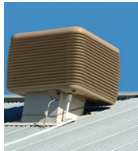
The main unit of an evaporative air-conditioner is usually located on the roof
