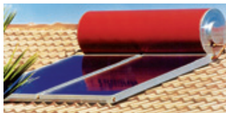
A solar hot water system will generally have solar collector panels on the roof
